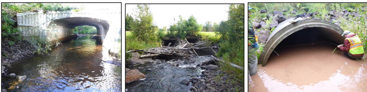
Figure 82: AOP Blockages: No blockage of W. Branch Knife River (left) and Significant blockages of left barrel of East Branch Beaver River (center) and Tributary to Saint Louis River (right)
