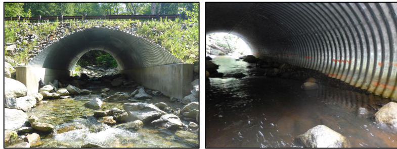
Figure 81: Bed instability: White River is Very Stable with no signs of bed movement (left); Pre-emption Creek is Very Unstable, the lower spray paint marker indicates original streambed elevation, higher spray paint marker indicates original interior bank elevation (right)
