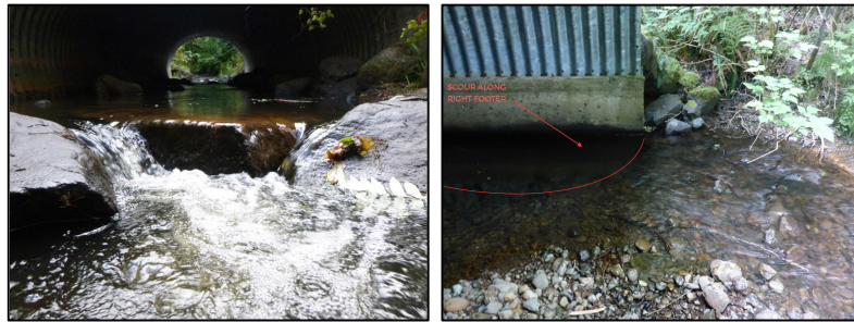
Figure 62. Scour hole downstream of rock sill at culvert exit at Pre-Emption Creek (left) and Observed scour at the entrance to Tributary to Schafer Creek (right)
